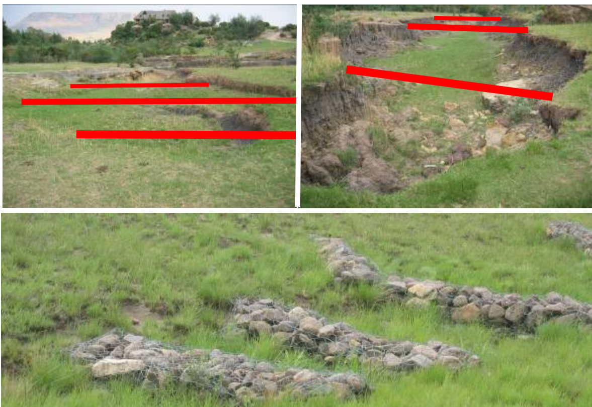
Figure 9a – where and how to stop the head of the gully from growing further uphill
